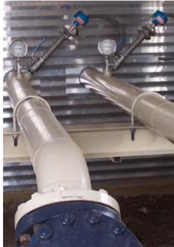
Natural gas flow at a gas production plant is monitored to provide flow measurement from each individual well. The main custody transfer meter is positioned downstream from where the flow from individual lines is combined.
