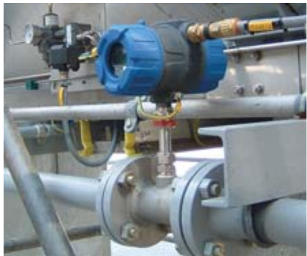
Measuring natural gas flow to a furnace. The use of an insertion probe permits the TA2 to be installed in lines of various sizes and with considerable installation flexibility while also ensuring economical mass flow measurement.
